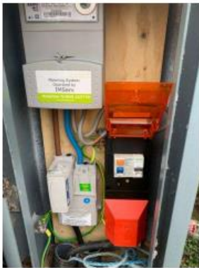
Meter installed within small feeder pillar
