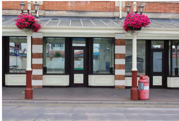
Appropriate traditional stall risers but dark brown joinery is out of character and mirrored glass would benefit from replacement with clear glass to create an active frontage
