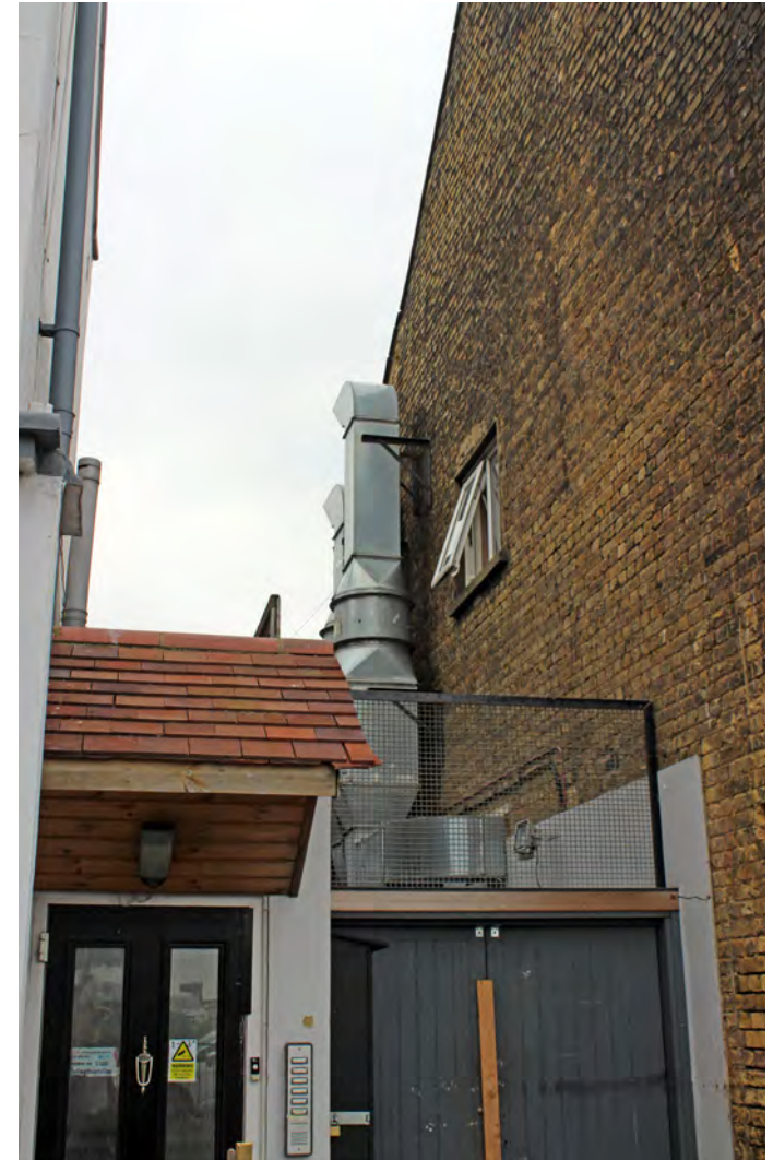
Unsightly ducts and modern entrance porch
