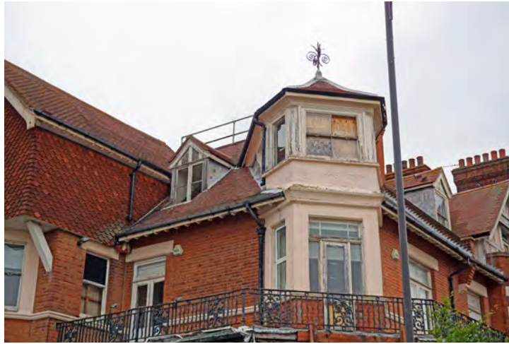
Poor condition of the former Beecroft Gallery (2019)
