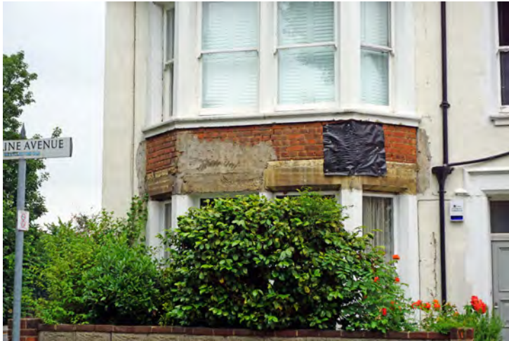
Poor condition of a bay window on Marine Avenue (2019)
