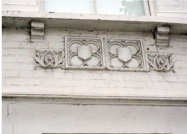
Brickwork and terracotta decorative tiles painted over (2019)
