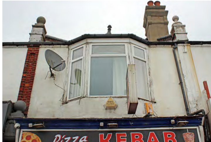
Inappropriate uPVC windows, burglar alarms, satellite dish and shop signage
