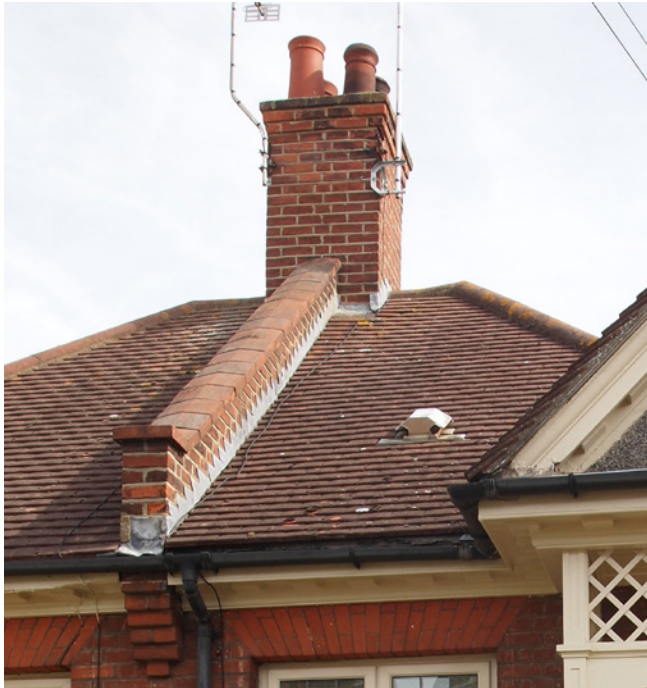
Detail of the roof showing stepped brick at the top of the chimney stack and corbel at the base of the ridges.
