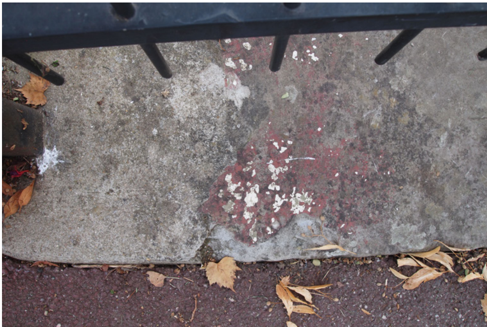
Remains of an existing path and red surface
