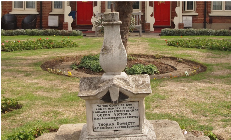
Leaning sundial with missing dial and in need of repairs to the base
