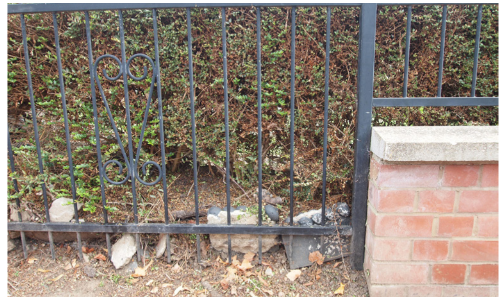
Dislodged edging tiles behind the front boundary railings
