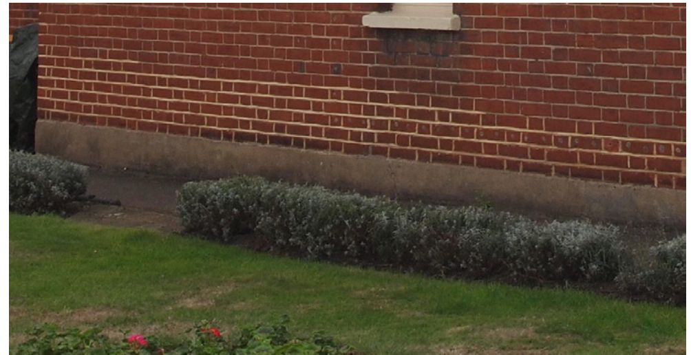
Small filled holes indicating an injected damp proof course
